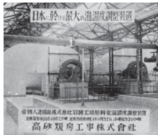
1927 Japan's first Precised temperature and humidity Control System (Iwakuni Plant of Teikoku Rayon Co., Ltd. (current Teijin Limited))
