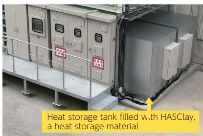
External view of a fixed heat storage system
