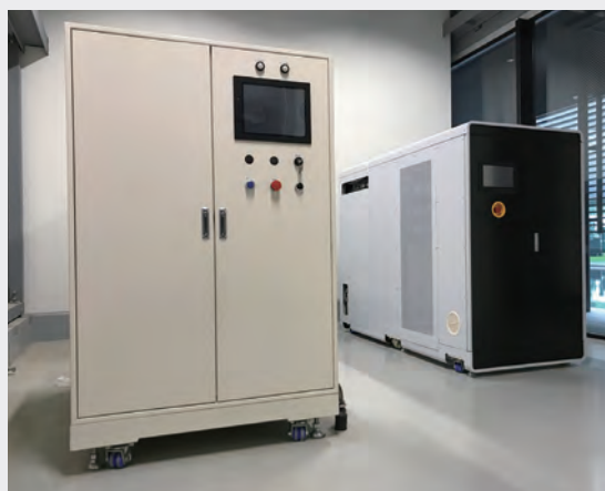
Hydrogen system exhibition room (Takasago Thermal Engineering Innovation Center)
