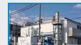
In-plant cogeneration system → Recovering heat from exhaust gas (160°C) and exhaust warm water (80°C)
