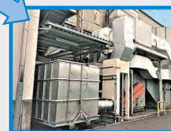
In-plant industrial air conditioning (painting process) → Reduction in dehumidification and heating load
