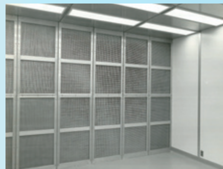
Takasago laminar flow cleanroom
