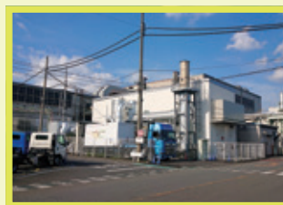
In-plant cogeneration system ▶ Recovering heat from exhaust gas (160°C) and exhaust warm water (80°C)
