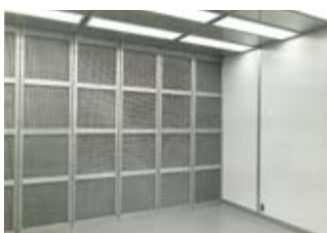
Takasago laminar flow cleanroom
